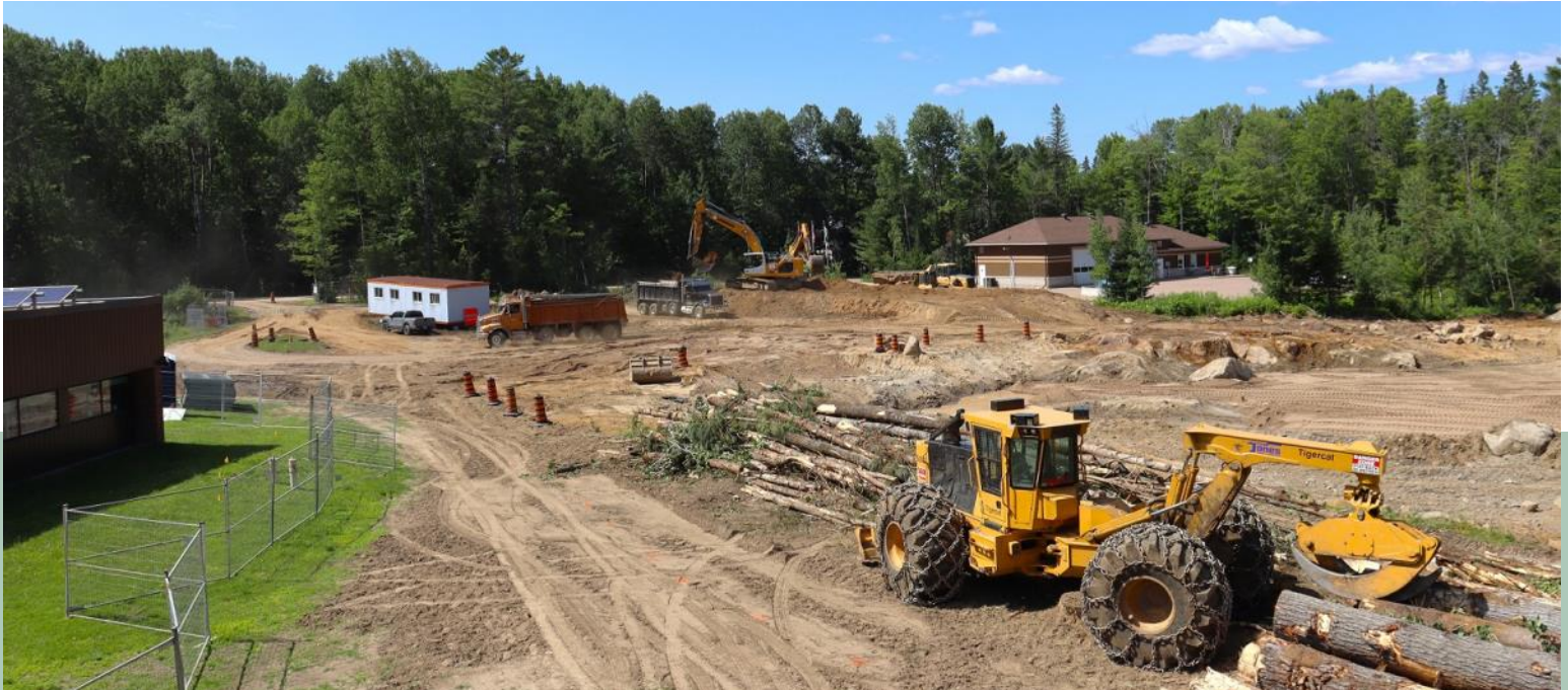
Pictured above is the build site of the new Four Seasons Lodge Long-Term Care Home at Deep River and District Health on July 11, 2024.
